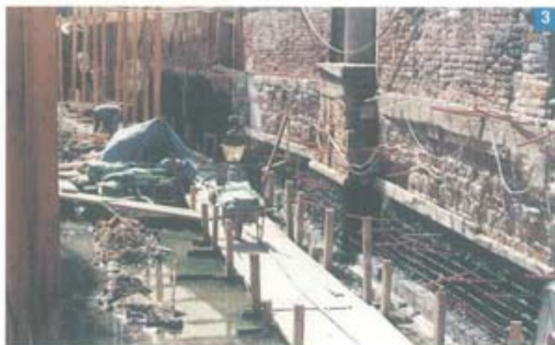
Photo 3. A dry canal. Stabilcem , a superfluid expanding cement binder used for filling cracks and cavities and porous gaps in rock and concrete, is injected into the canal bank. The product has here been used in the HV (high viscosity) version, specially developed for this building work.
