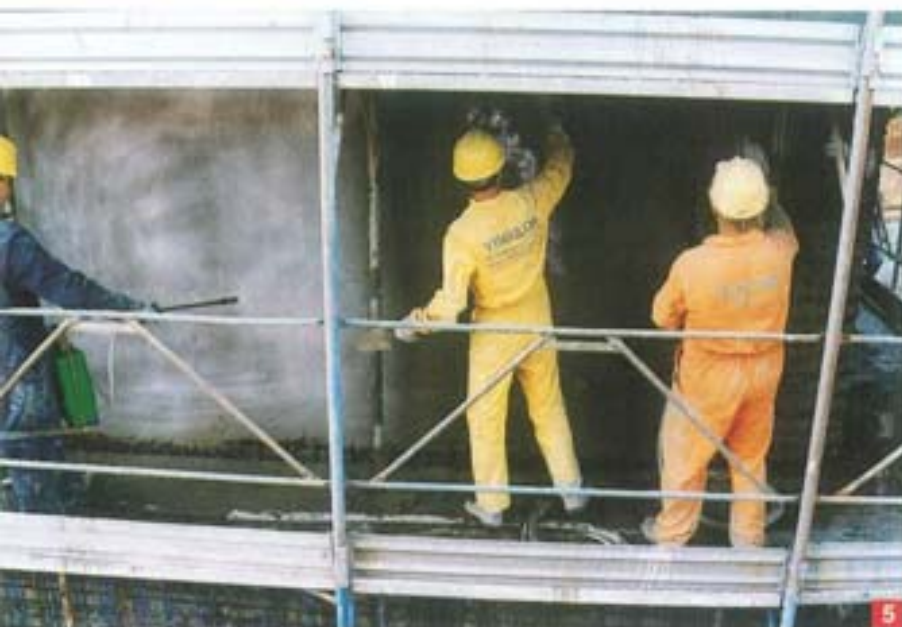
Photo 1. Close-up of degraded concrete
