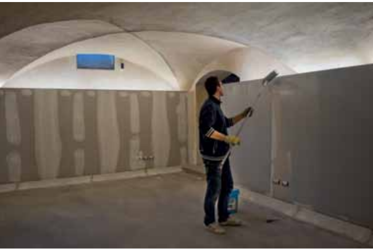
ABOVE. The walls were primed with tinted QUARZOLITE BASE COAT (left) and then painted with QUARZOLITE PAINT (right).
