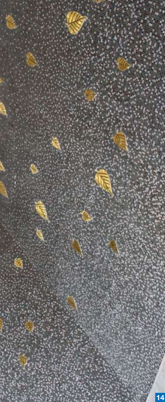
Photo 14. View of the mosaics featuring the shape of pho leaves, which were made in different sizes and bonded with ADESILEX P10+ISOLASTIC on a total of 8 panels on inside walls.
