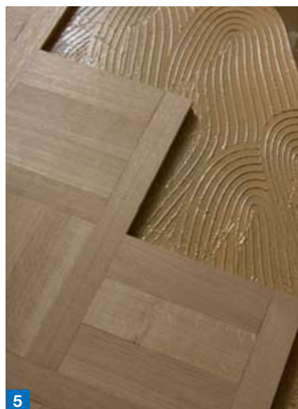
Photo 1. Heidelberg City Hall is located in the centre of this ancient German city. On the second floor wooden floorings were laid with Mapei products.
