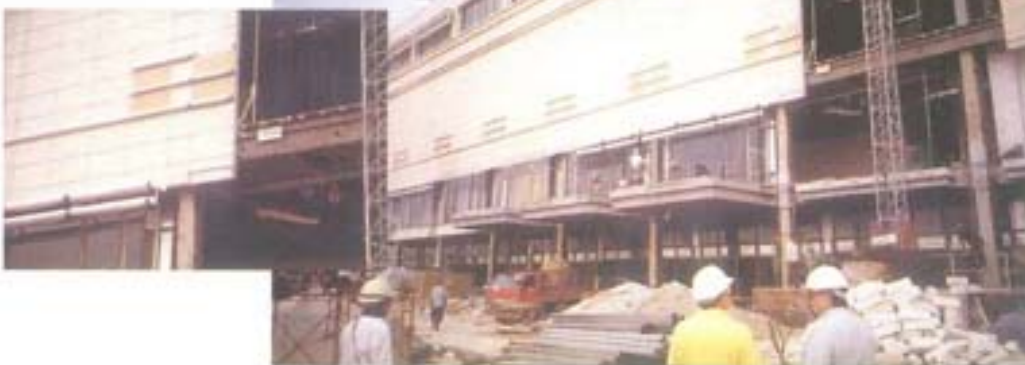
Work in progress Right: cladding the exterior of the Suria KLCC Centre (with detail)
