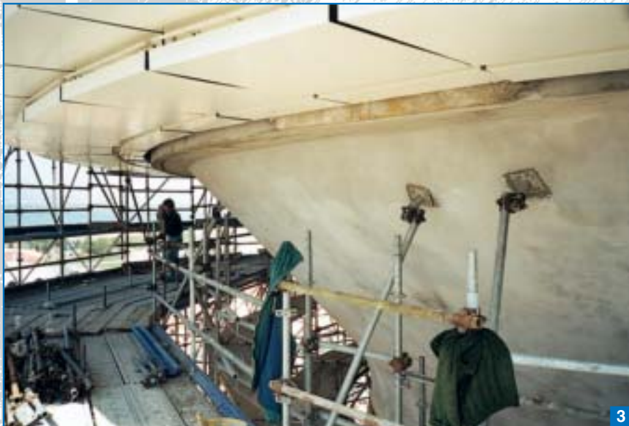
Photo 3. Application of the coating layer on the deteriorated areas with NIVOPLAN F*.
