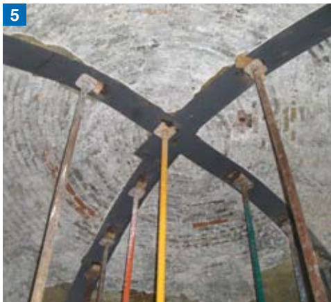
Photo 5. A detail view of the temporary support used for the vaulted roof to avoid it collapsing.
