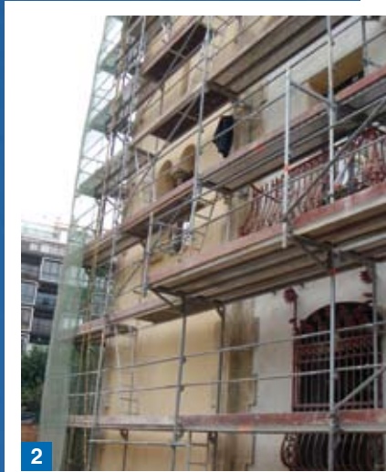
Photo 1. The state of deterioration and abandonment in which Villa Florida was to be found prior to the restoration work.
