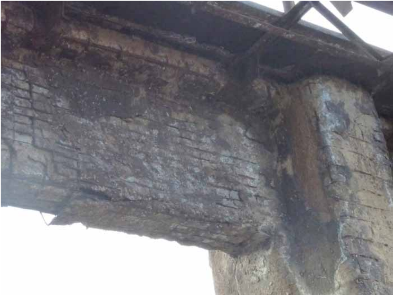
Zone I. Crane beams degradation.
