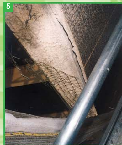
Photo 5. Partial detachment of the installation mortar from the underlying levelling concrete without the collapse of the glass mosaic.
