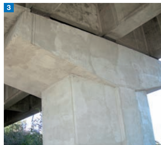
Photo 4. ELASTOCOLOR PRIMER and ELASTOCOLOR PAINT were used for the final protective coat.
