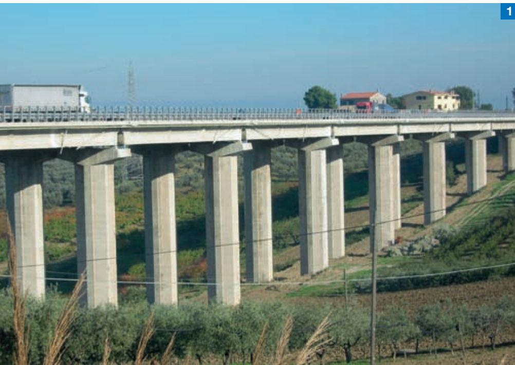
Photo 1. An image of the Ilde viaduct before repair work.
