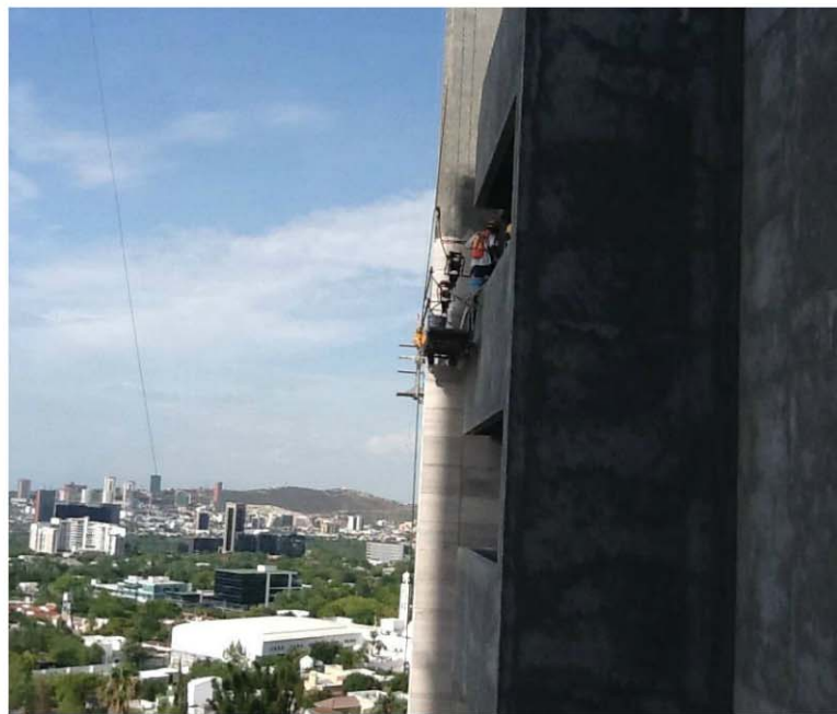
Using Ultraflex LFT from Mapei of Deerfield Beach, FL, allowed the installers to create a smooth flush look to the tiles all along the installation.
