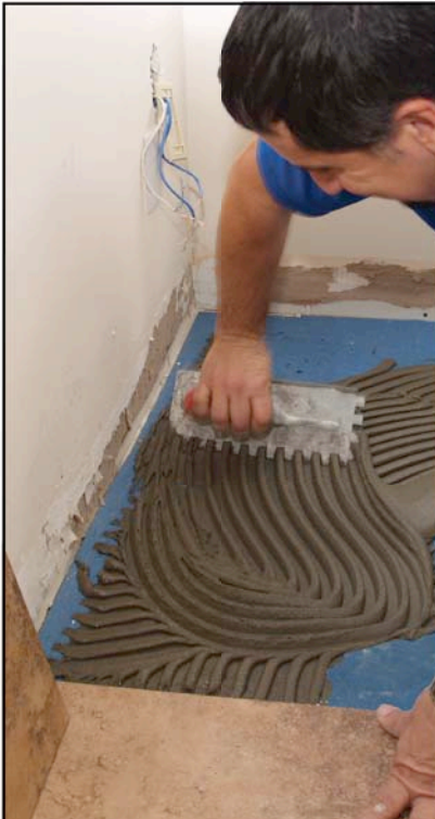
Granirapid flexible mortar system was used to install 20,000 sq. ft. (1,858 m 2 ) of porcelain tile on the building's upper level.
