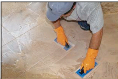
Kerapoxy chemical and stain-resistant grout was used to grout 35,000 sq. ft. (3,252 m 2 ) of porcelain tile throughout the building.
