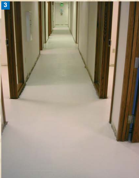
Photo 1. This one-storey structure was built into a hillside, which caused its floorings to be deeply damaged by humidity.
