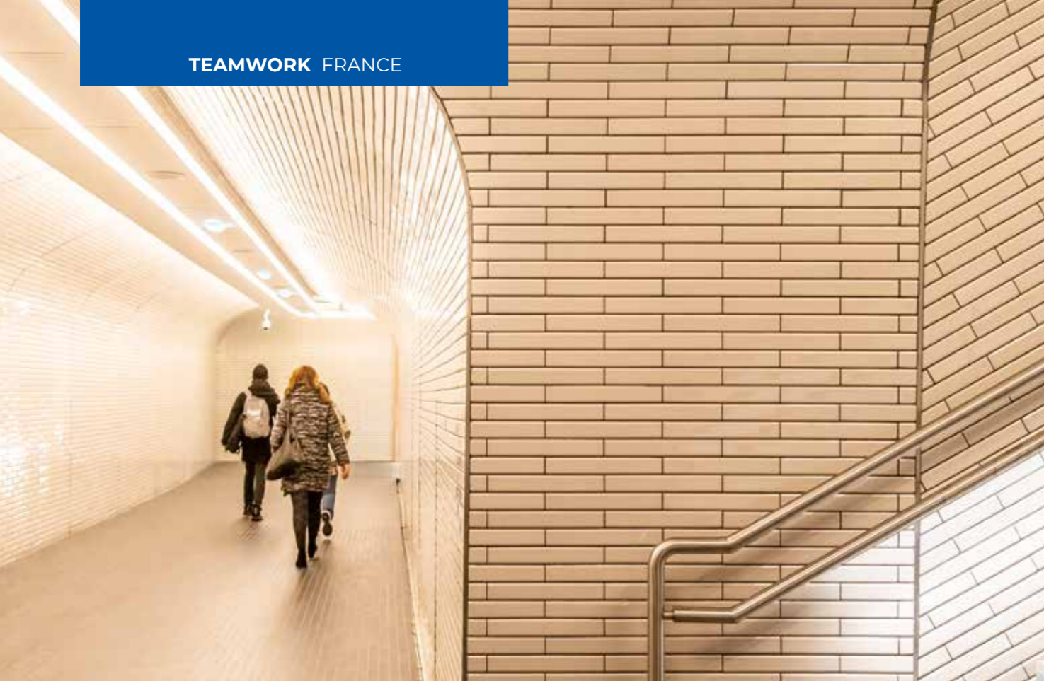
Ceramic floor and wall tiles were installed in the new stations along Line 14 using Mapei products such as GRANIRAPID, KERALASTIC T, ULTRALITE S2 QUICK and ULTRACOLOR PLUS.
