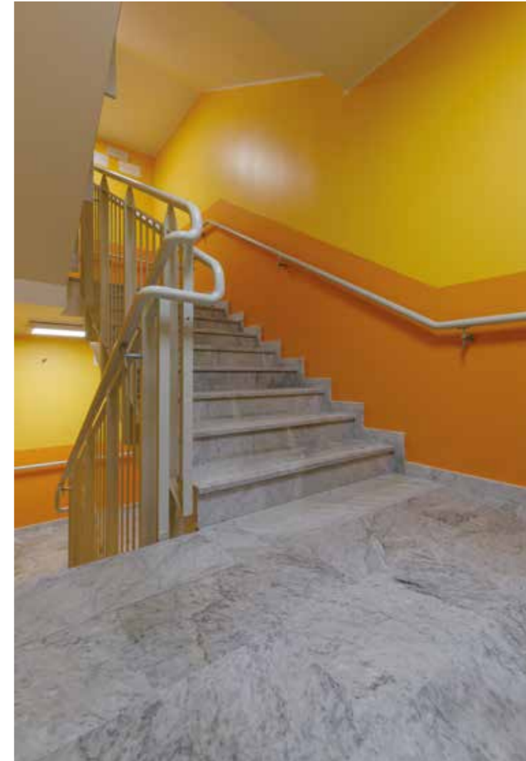
Stone coverings were installed on the stairs and landings in the service areas with ADESILEX P9 EXPRESS.
