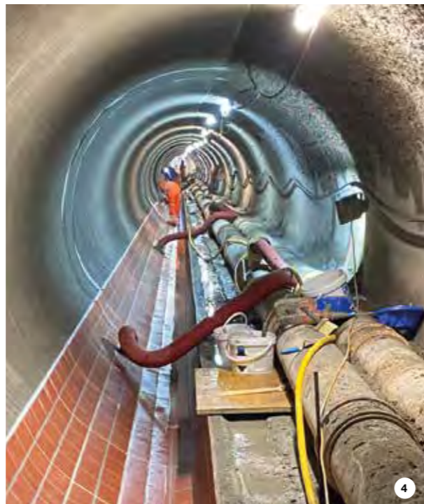
3. To guarantee the waterproofing capacity of the expansion joints, MAPEBAND FLEXROLL membrane is being applied and bonded in place with ADESILEX PG4.
