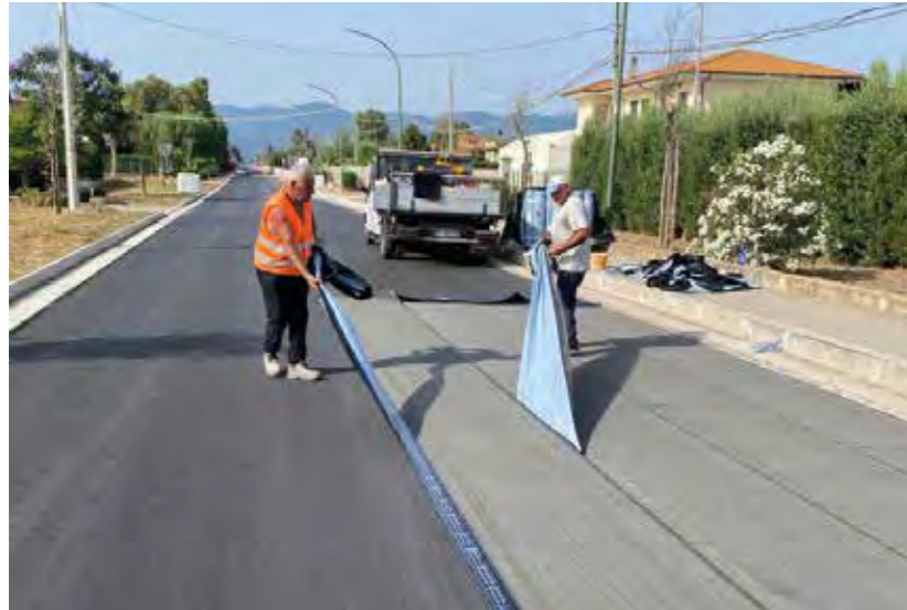
TOP OF THE PAGE, LEFT. Installing POLYSTRADA SA membrane on the road surface.
