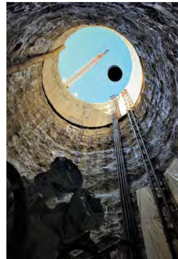
IN THE FACING PAGE. The 3RPORT project includes a deep rock tunnel to collect and convey Combined Sewer Overflows (CSOs) from 22 outfalls along the St. Marys and Maumee Rivers. ABOVE. One of the shafts included in the 3RPORT project.
