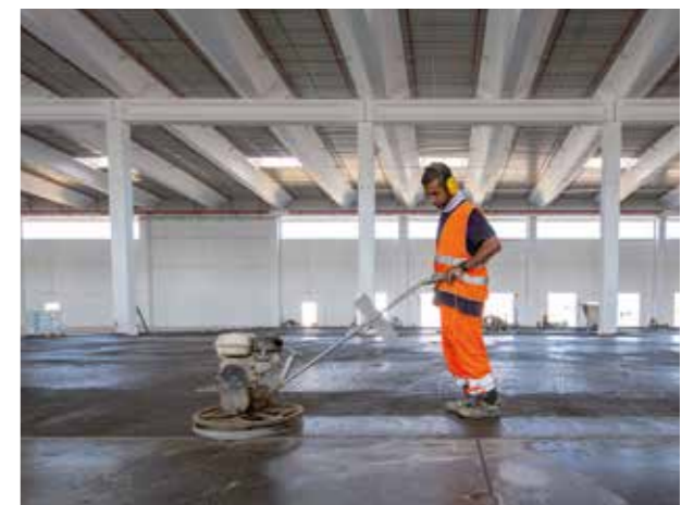
MAPETOP N AR6 and MAPECRETE LI HARDENER were used to finish the floors, before smoothing them with "helicopter" power trowel.
