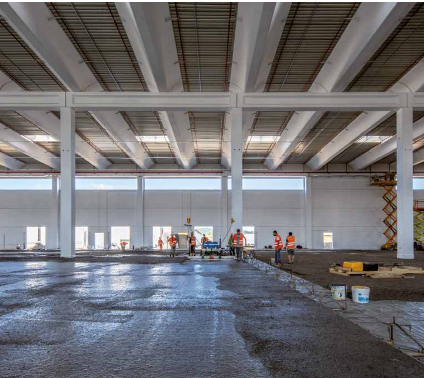
MAPEFIBRE ST 50 TWISTED macro structural fibers and the acrylic-based superplasticiser DYNAMON FLOOR 20 were added to the concrete mix used to make the floors.
