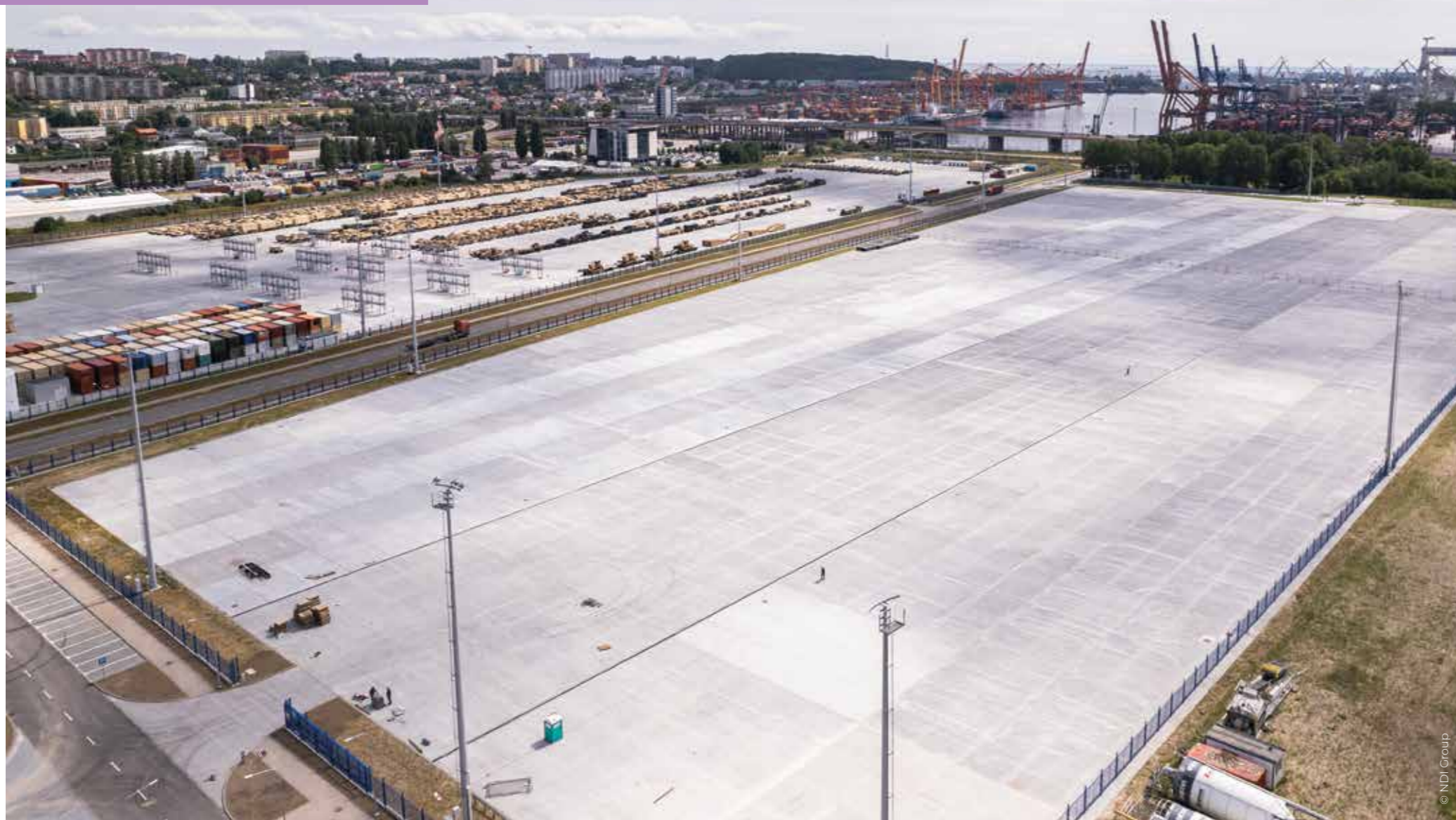
LEFT. Storage yards covering an area of 18.6 hectares were constructed in the Port of Gdynia. Concrete floors were completed with Mapei fibers and admixtures.
