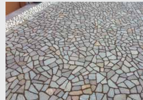
Paving made from assorted sizes of recovered cobblestones, cubes and irregular stone units sealed with MAPESTONE JOINT.
