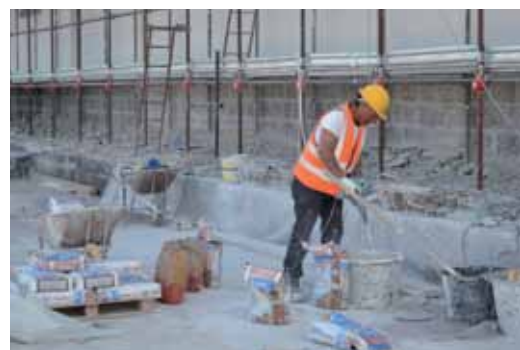
The façades of the 7 workshops were renovated using solutions from the MAPE-ANTIQUE line.
