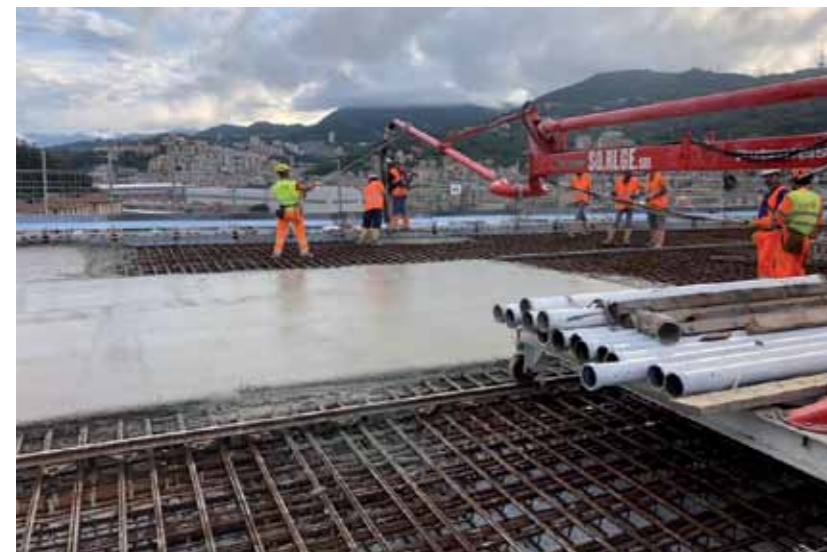
DYNAMON XTEND W202 N, DYNAMON LZ 551 and EXPANCRETE PLUS admixtures were supplied for the concrete poured on the deck.
