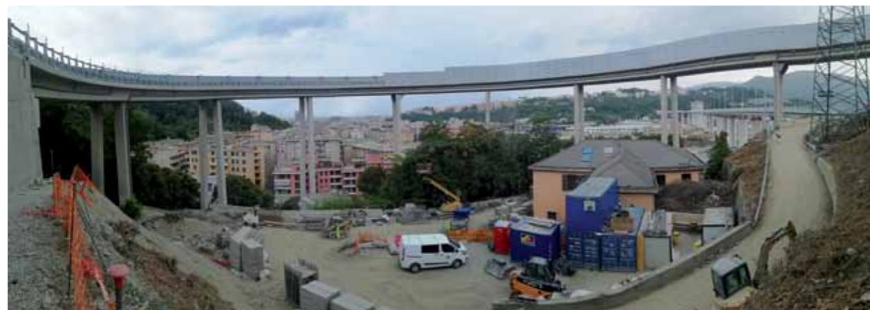
ABOVE. Repair work was carried out on both the intrados and the extrados of the bridge deck. Various products by Mapei were used for the job, including MAPEGROUT EASY FLOW fibre-reinforced thixotropic mortar and the hi-flow mortars MAPEGROUT GF BETONCINO B1 and MAPEGROUT HI-FLOW B2.
