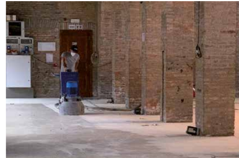
RIGHT. Before applying MAPEFLOOR SYSTEM 33 for resin floors, the substrates were grinded with a diamond grinding disk.
