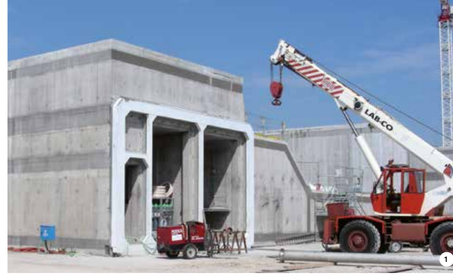
1. Reinforced concrete caissons used in the Mose project during their manufacture. The joint housings for the caissons were connected together with a jointing system made up with MAPEFILL MF 610.
