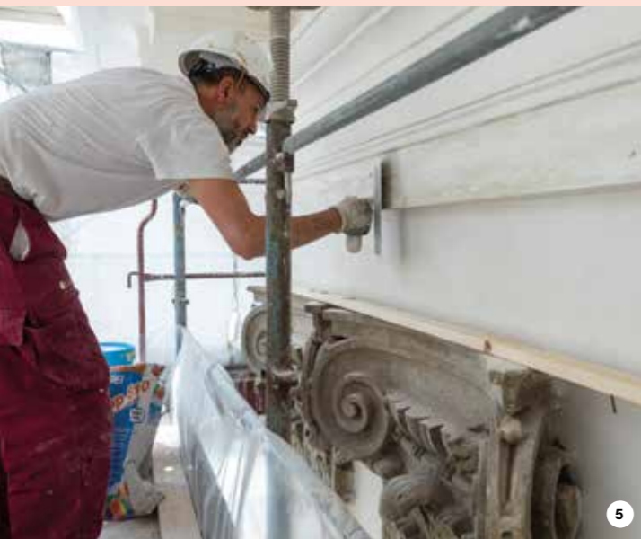
5. PLANITOP 510 fine-textured, lime-cement skimming mortar was applied on the external surfaces before painting them. When the render was made of lime, the product chosen was MAPE-ANTIQUÉ NHL ECO RASANTE CIVILE fine-grained, breathable, smoothing and levelling mortar.
