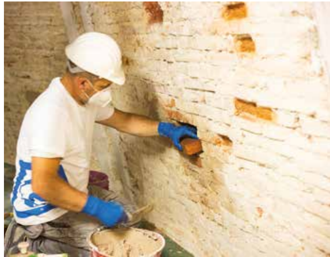
LEFT. The gaps and voids from the putlog holes were repaired by filling and plugging them with the original bricks and MAPE-ANTIQUE ALLETTAMENTO.
