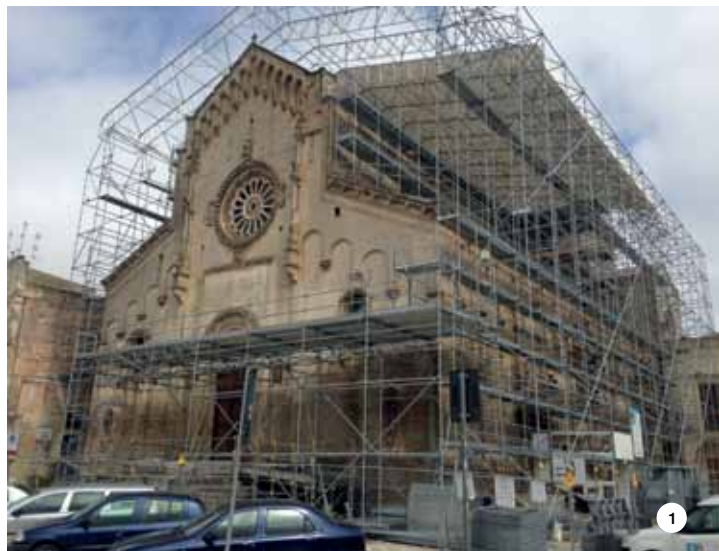
PHOTO 1. The MAPEWOOD system was used for the wooden roof beams and trusses and the MAPEWRAP system was applied to strengthen the structure.
