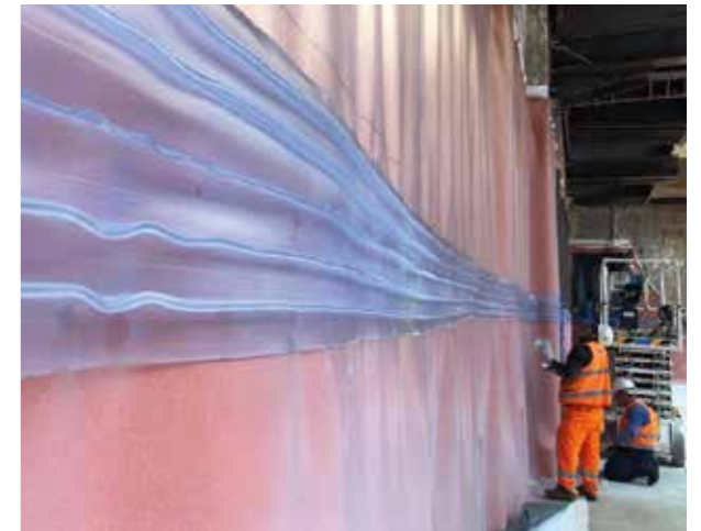
ABOVE. The Mapei Group supplied concrete admixtures and waterproofing membranes for the M4 line.
