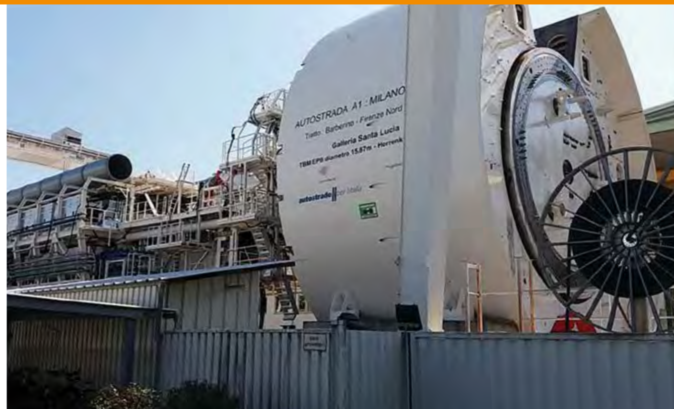
ABOVE. With a diameter of 15.87 m, the TBM used for the Santa Lucia tunnel was the largest tunnel boring machine ever used in Europe at the beginning of the works.
