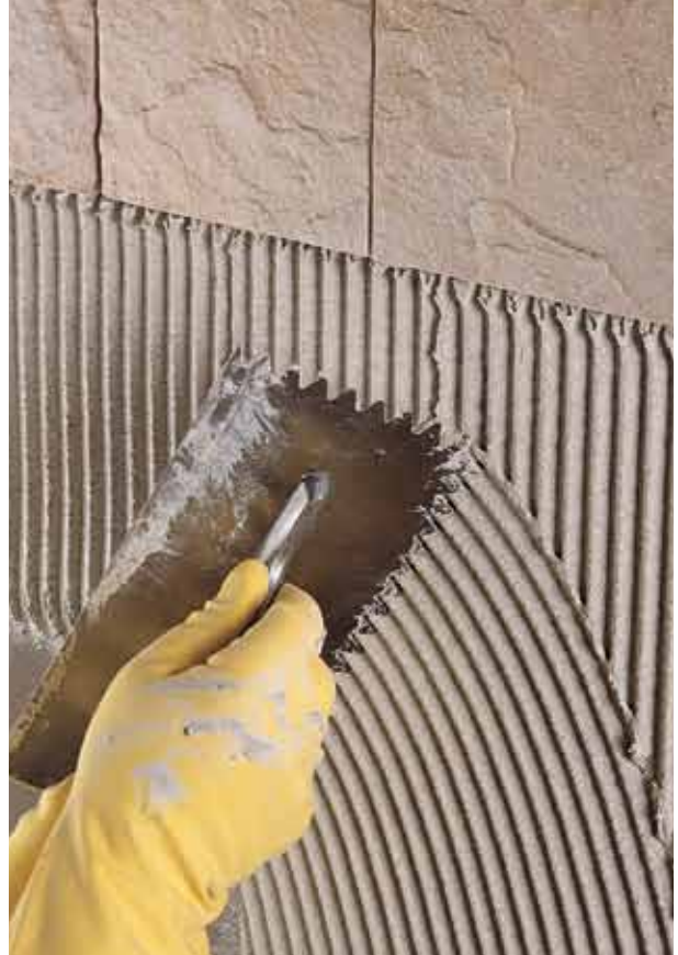
ADESILEX P9 was used to bond porcelain tiles on both horizontal and vertical surfaces
