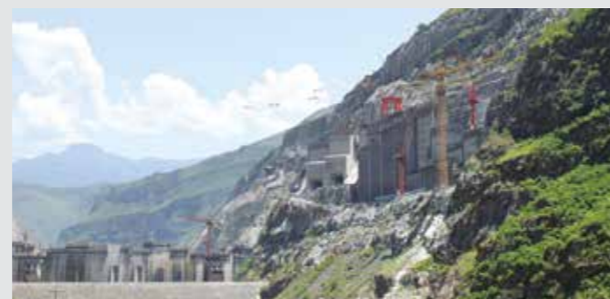
XILUODU HYDROPOWER PLANT Xilodu, Yunnan Province - China
