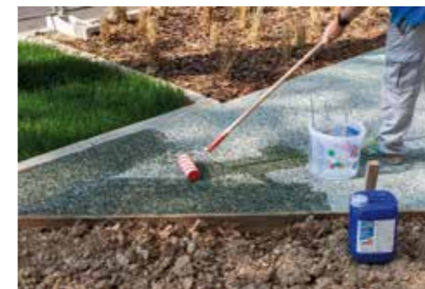
Products from the Mapei Color Paving® system were used to create the decorative concrete platforms (left). PLANISEAL WR 100 (right) ensured hydrophobising protection for the fountain.
