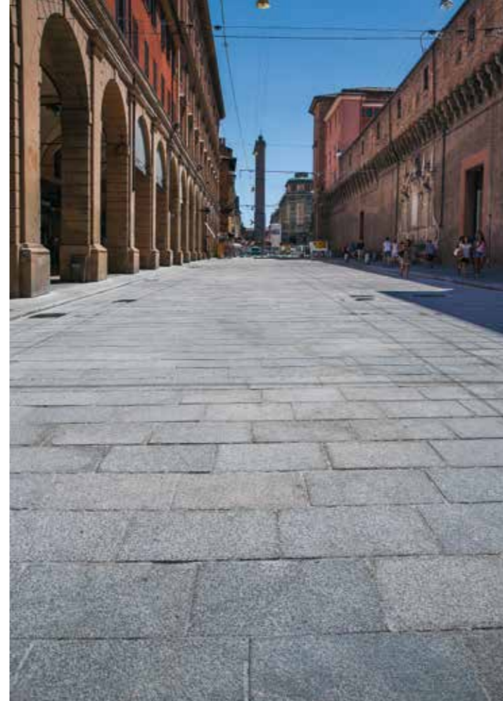
The paving of Strada Maggiore in Bologna was renovated in 2014 by using MAPESTONE TFB 60 mortar.
