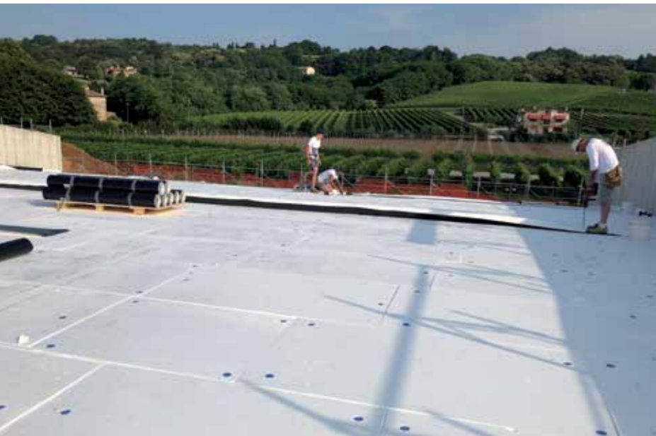
ABOVE. Application of Mapeplan T B synthetic membrane over the insulating layers.
