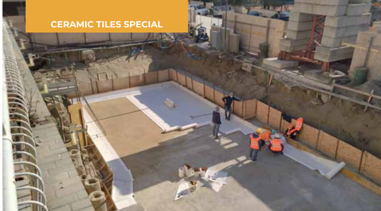
Underneath the storage tanks, the foundations were waterproofed from under the slab with MAPEPROOF FBT, a waterproofing membrane made up of a synthetic FPO sheet tightly coupled to a layer of non-woven fabric.
