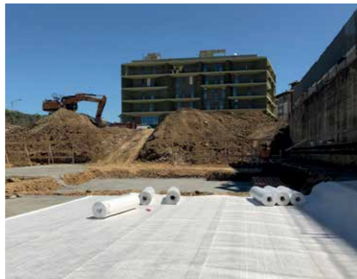
A view of a building site where Mapei fully-bonded waterproofing membranes were used.
