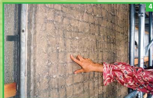
Photo 4. Complete detachment of the installation mortar and, therefore, of the glass covering leaving the levelling concrete visible.
