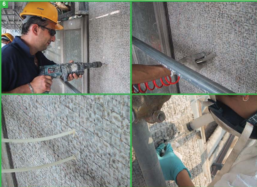
Photo 6. Injection of Epojet LV epoxy resin. Drilling the injection holes (diameter of the holes: 10 mm; depth: 30 mm) in order to intercept the gap between the installation mortar and the levelling concrete. Cleaning the holes with compressed air. Positioning the injection tube and the monitor tube into the holes. Injecting epoxy resin.
