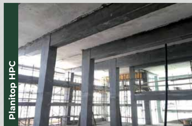
Strengthening by jacketing reinforced concrete pillars, beams and beam-pillar joints with compact layers of PLANITOP HPC.
