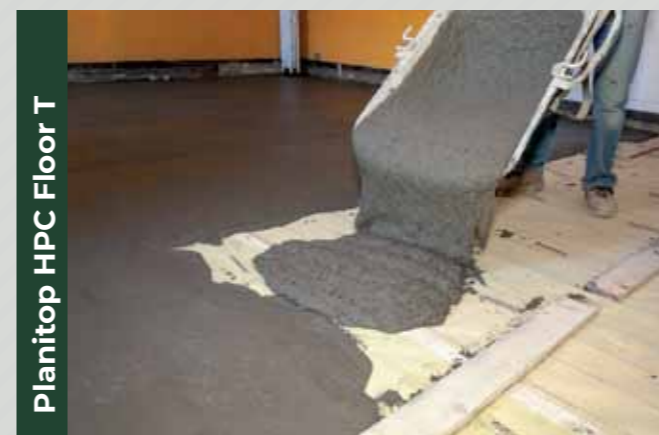
Strengthening of the extrados of wooden slabs with a low thickness structural screed realized with PLANITOP HPC FLOOR T.
