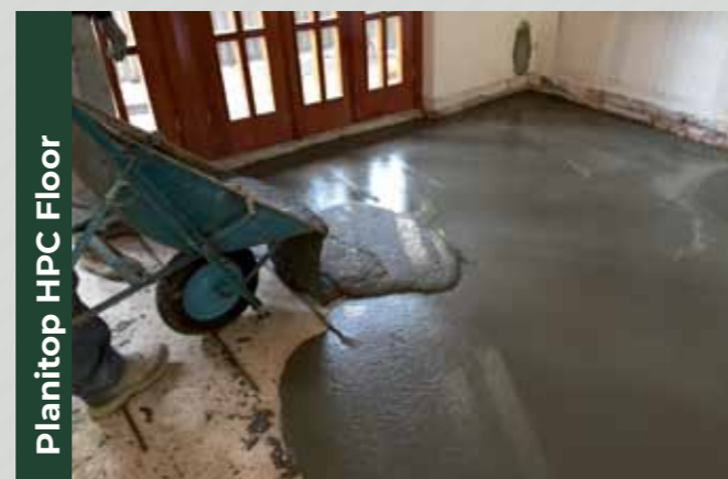
Strengthening of the extrados of a brick-concrete slab with a compact layer of PLANITOP HPC FLOOR.
