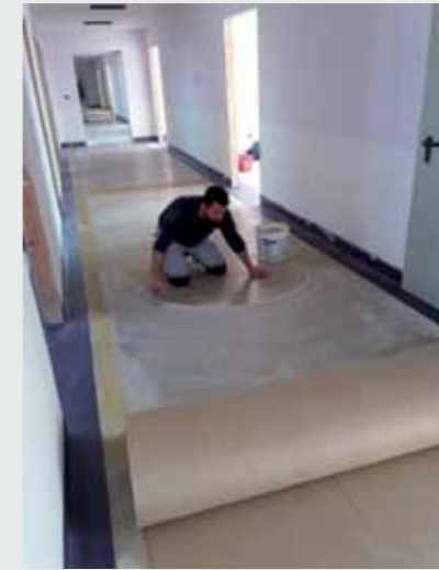
Installing floors with Mapei products. LEFT. Madonna Delle Grazie Hospital in Matera (Southern Italy). RIGHT. Don Tonino Bello Hospital Molfetta (Bari), Southern Italy.
