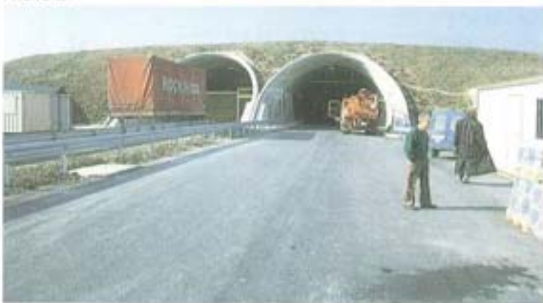
PHOTO 12 and 13 The entrance of the two tunnels at an initial stage and once finished
