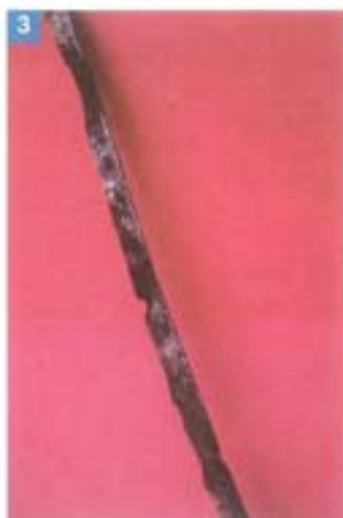
Photo 4. Corrosion due to carbonization and presence of chlorides.
