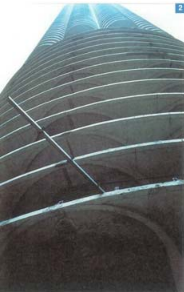
Photo 1. A skyscraper in Boston, showing signs of corrosion due to carbonization.
