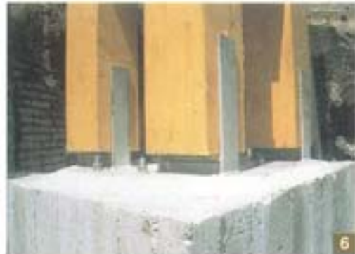
Photos 5 and 6 - New concrete bases were placed over the original stone blocks. The wooden beams were then placed on top of the concrete.
