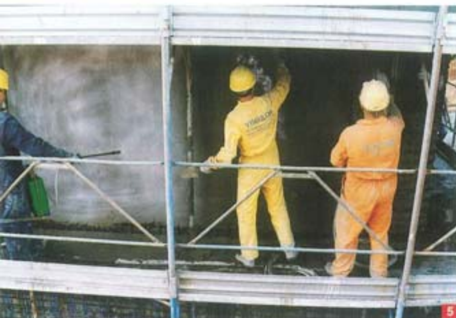
Photo 1. Close-up of degraded concrete
