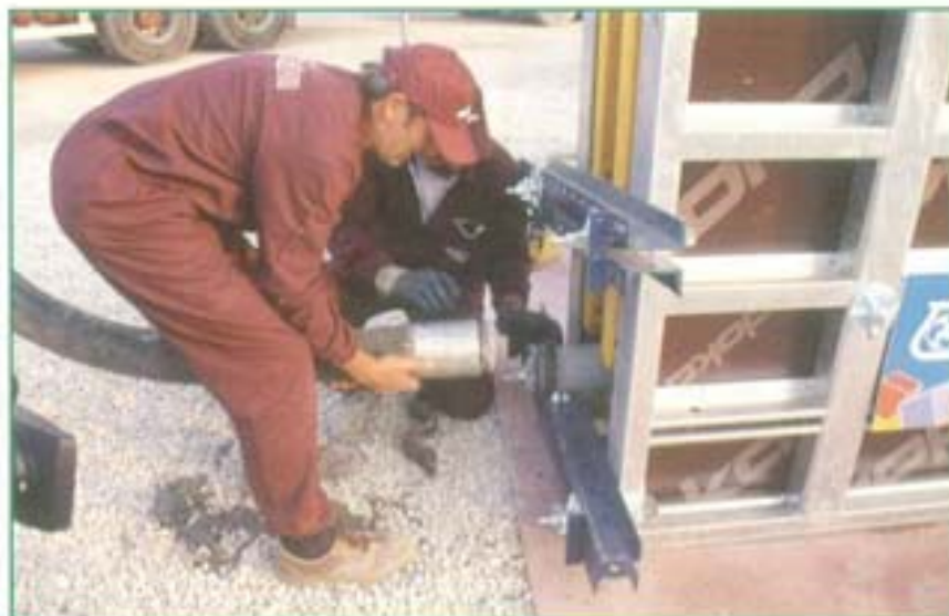
Fig. 7. Construction of a supporting wall by casting of self-compacting concrete from the bottom.
