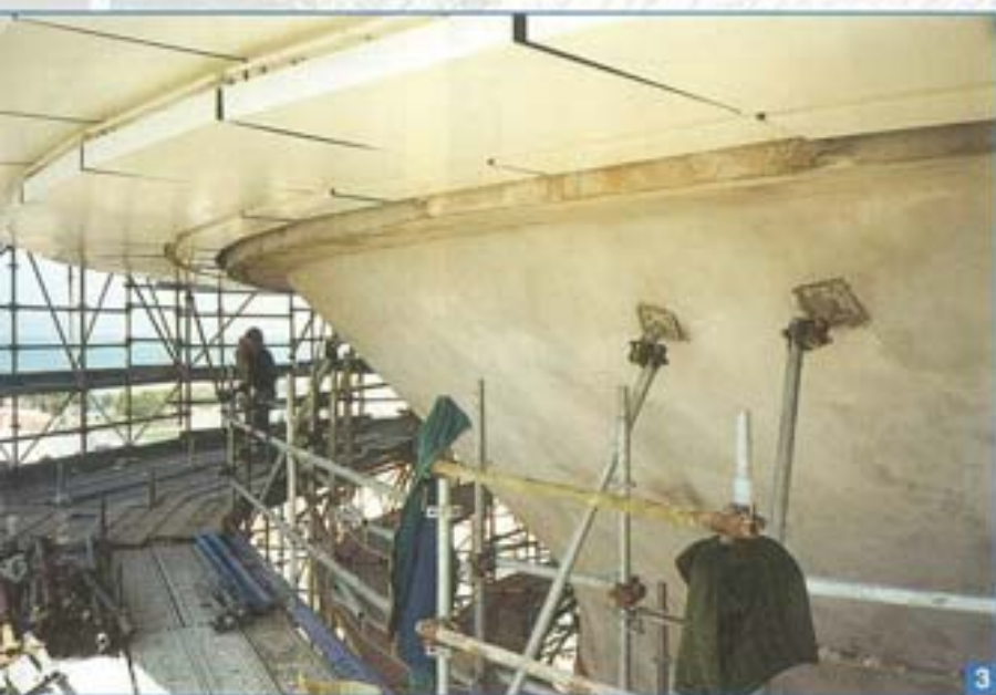
Photo 3. Application of the coating layer on the deteriorated areas with NIVOPLAN F*.
