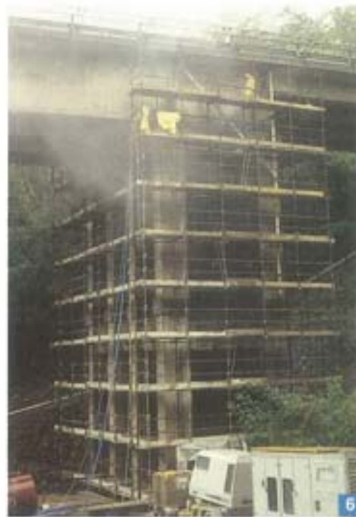
Photo 5. Detail of the deterioration of the viaducts structures. In particular, the emerging of the rods and their corrosion are evident.
