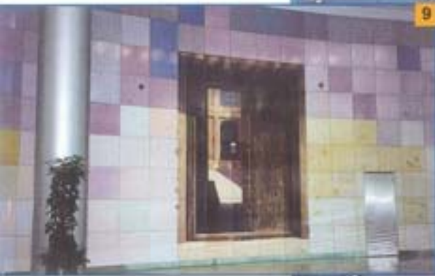
Photo 9. A detail of the access corridors to the lounges and hotel: large-sized ceramic tiles (60x60) were used and installed with KERACRETE.
