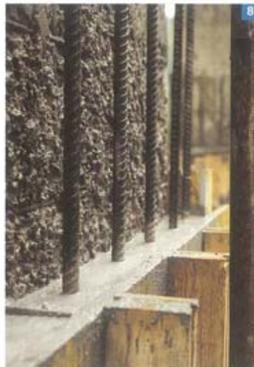
Photo 7. Detail of the consolidation and integration intervention (a new layer of concrete was applied) of the base of the viaduct piers using concrete with compensated shrinkage, carried out according to the above described procedures
