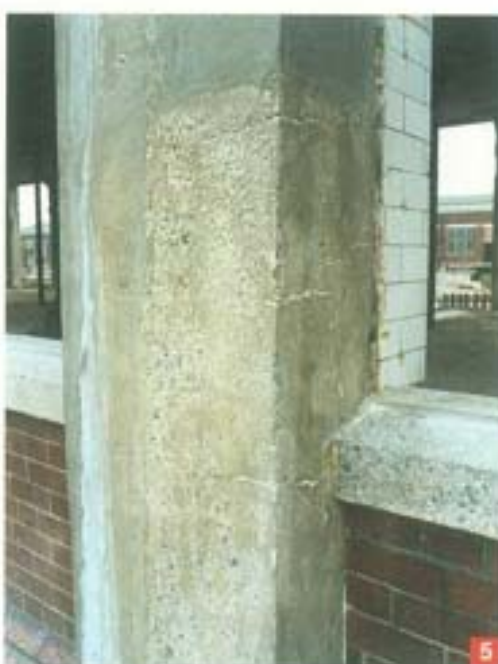
Photo 5. The structure of this column was reinstated with MAPEGROUT after repairing the steel.
