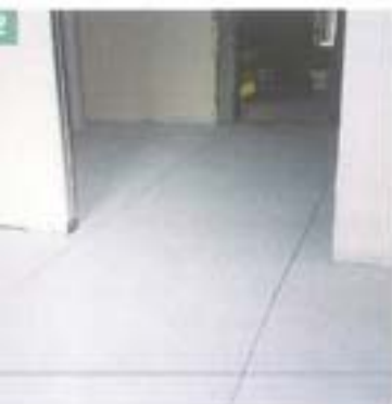
Photo 2. All the floor screeds were realized in cement and polystyrene hardened superficially with the water consolidating compound PROSFAS.
