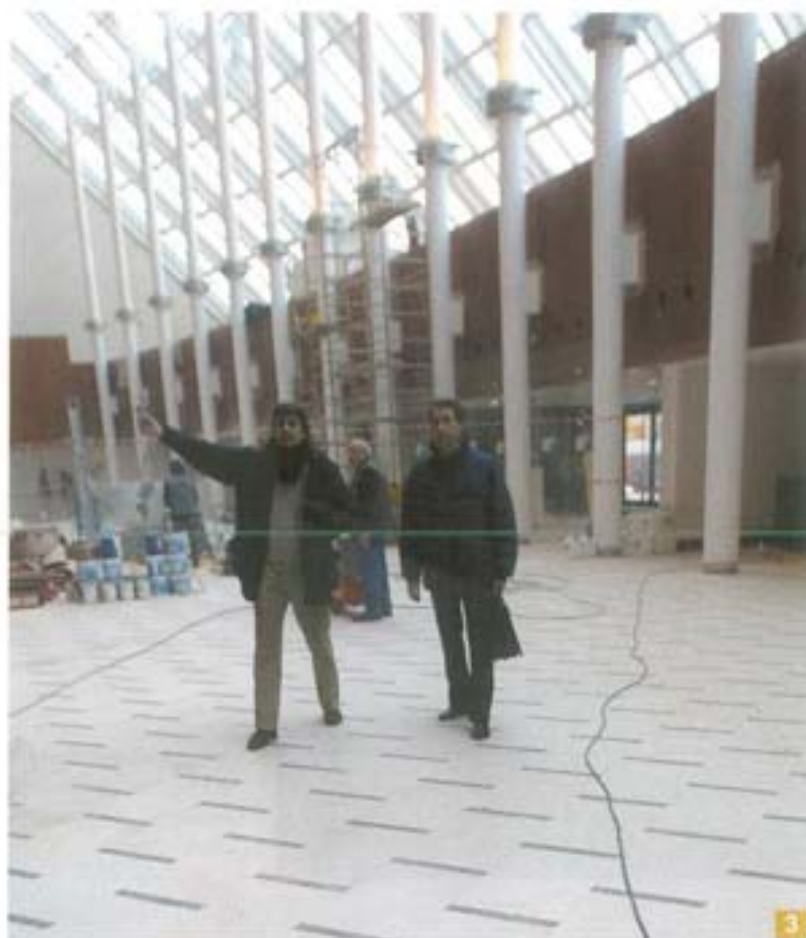
Photo 3. In the large atrium some bags of Nivorapid wait to be used for the levelling of the internal surfaces.
