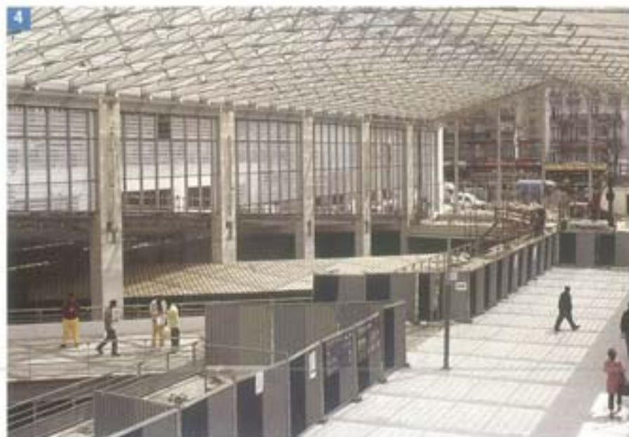
Photo 5. Thanks to its adhesive and quick drying characteristics, Granirapid allowed for the immediate placing into service of the flooring: it is, in fact, set to light foot traffic after only 24 hours.
