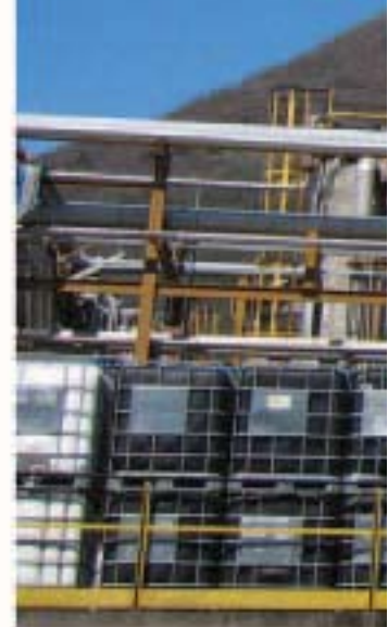
The Vinavil facility in Villadossola (VB) encloses a wastewater recycling system.
