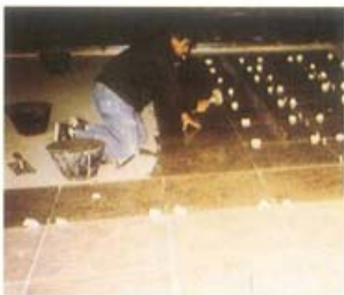
Three project stages : here below, mixing the two components of GRANIRAPID. At the center, installing the red granite from Madagascar (60X60X2 cm) with GRANIRAPID. At the bottom, after positioning, the granite slabs are tamped to achieve a proper adhesion of the back.
