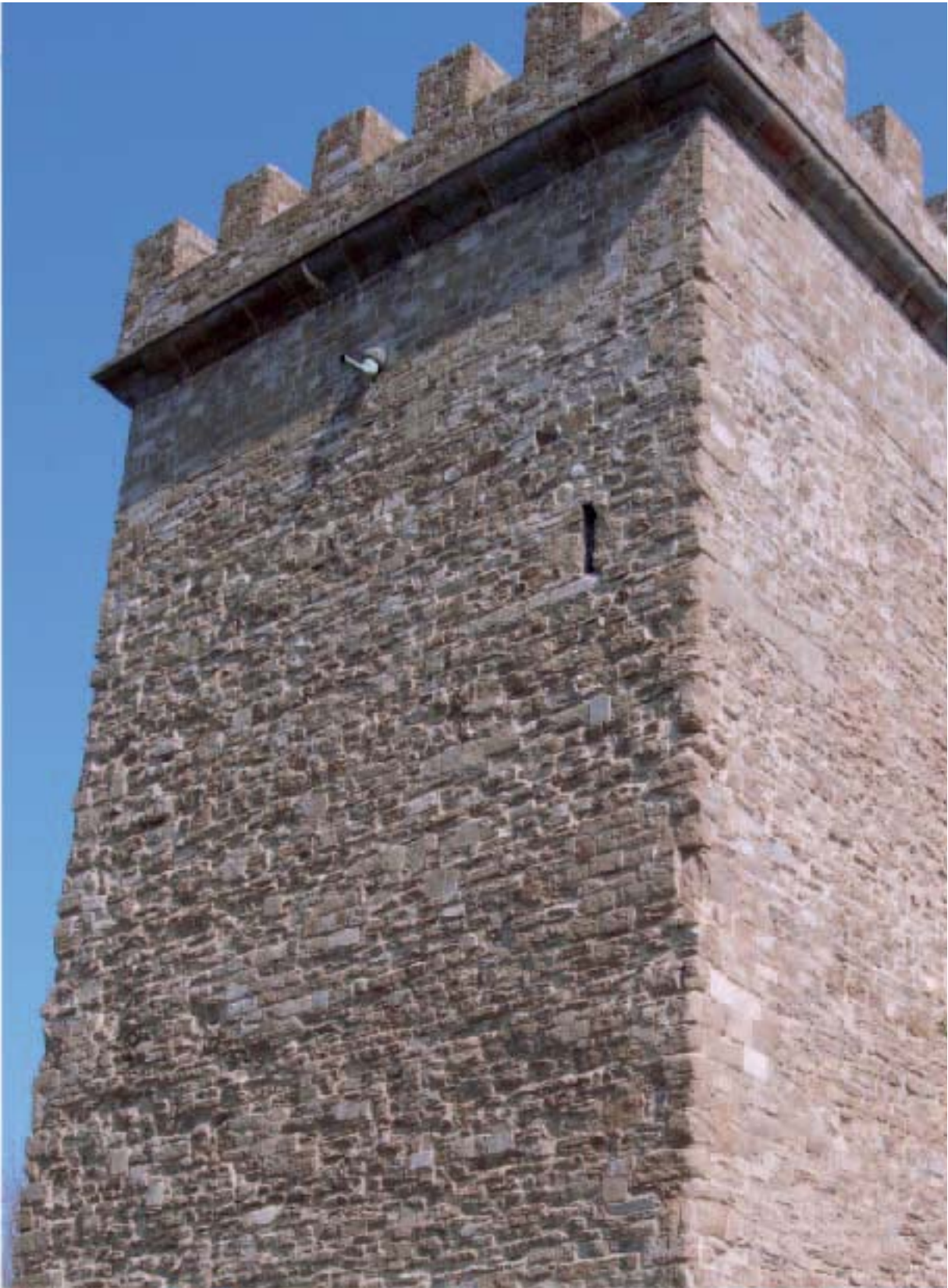
Photo 1 (previous page). Two pictures of the old Florence walls after renovation, which restored them to their ancient beauty. The work was carried out on the section of walls between Porta San Frediano and the Torrino di Verzaia.
