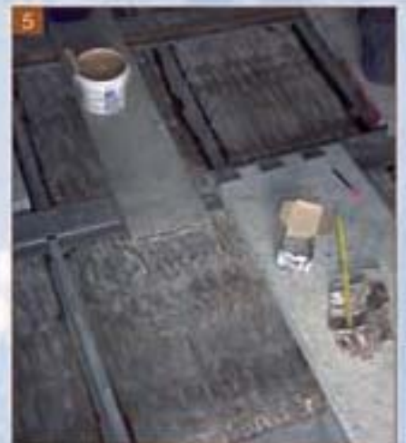
Photo 5. The reed mat ceilings in the Gothic Hall and the Chamber of Venus were consolidated on the outside with Eporip, used to bond the steel strengthening plates to the old wooden slats.
