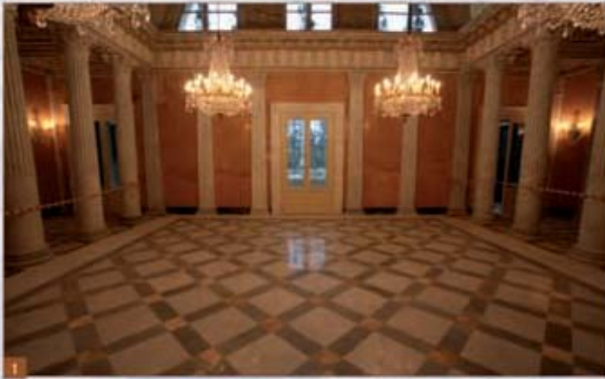
Photos 1 and 2. The floor screeds in the Ball Hall, with an incorporated heating system, were prepared with Topcem hydraulic binder. The marble slabs were bonded to the substrate using Granirapid adhesive.
