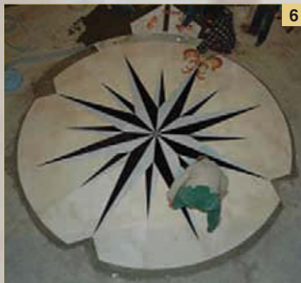
Photo 3. Before laying the star-shaped floor design, a screed was prepared with Mapecem on a substrate treated with a Planicrete-based bonding slurry.
