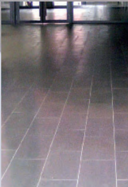
Ceramic tiles were laid with Mapei products in several inside areas of the stadium.
